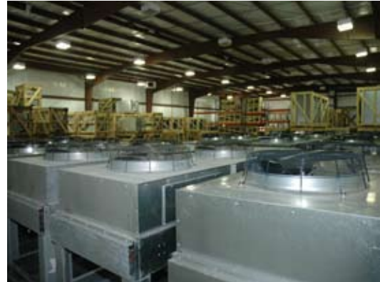
NEW REFRIGERATION EQUIPMENT
